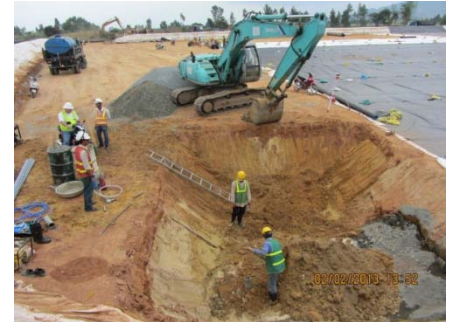
Constructing the sump in the drying pad to capture water (Photo: CDM Smith)
