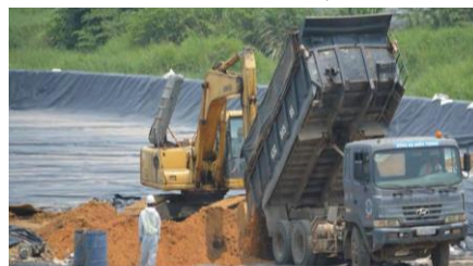
Placing Phase 2 contaminated soil in the temporary soil storage area (Photo: CDM Smith)
