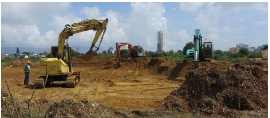
Clearing and grading the thermal desorption treatment pile area (Photo: CDM Smith)
